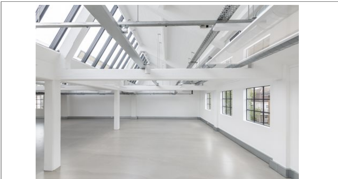
High-specification rooflights to newly-refurbished Gramophone Works included many features, such as non-fragility to CWCT Class 2, solar control glazing with G-Value of 0.38 and spread of ratings to BS 4761.
