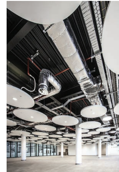
Ansty Park, Coventry Pendock Linea Ceiling Rafts
