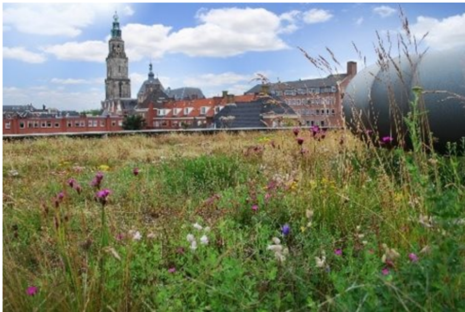
A blue roof is designed to store a large amount of rainwater for a given period of time and then release it slowly into the local surface water drainage system
