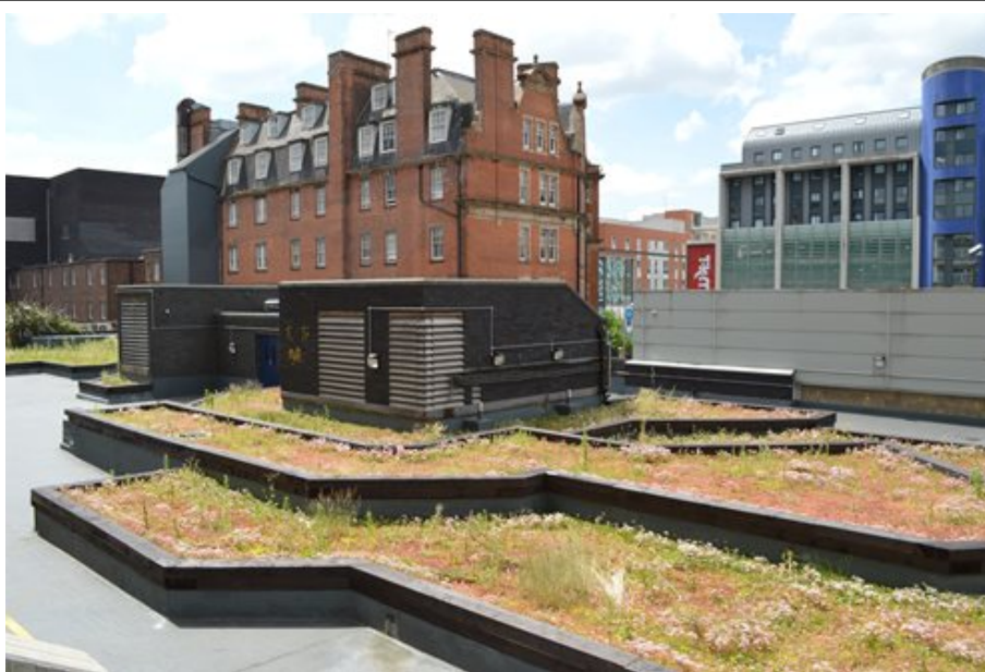
Victoria shopping centre, Nottingham: A blue roof solution was chosen to maximise rainwater retention and control water run-off during heavy rainfall conditions
