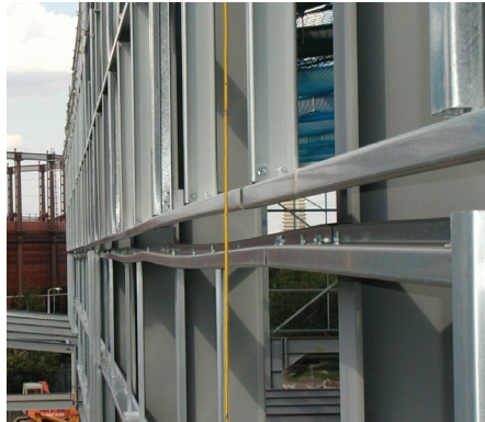
Poorly installed secondary steelwork.
