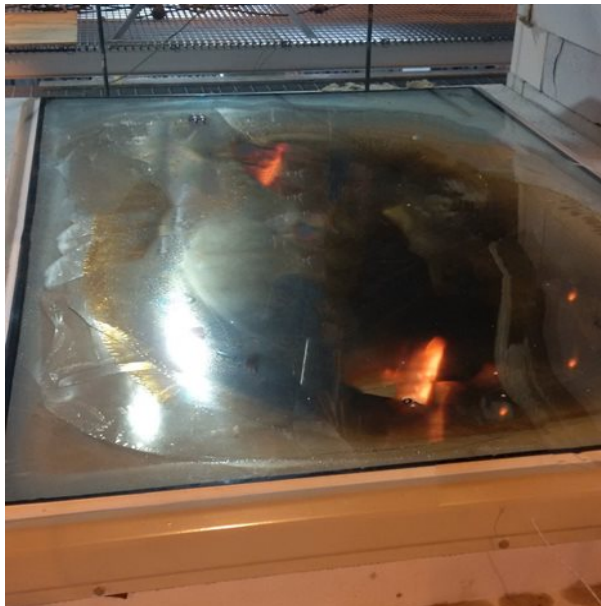
Rooflights are part of the building fabric and therefore they must match the fire resistant capabilities of the building elements.
