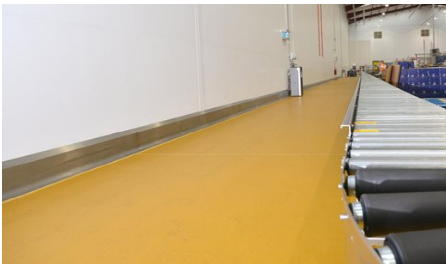
Polyurethane resin floor screed installed at 9mm thickness in a food factory
