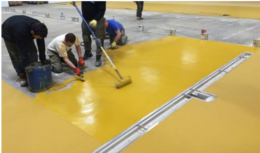
Polyurethane resin floor screed being installed by trowel and then lightly back rolled which helps achieve a consistent resin rich finish
