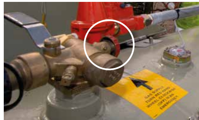
B. Above-ground tank gas isolation valve - Red hand-wheel circled above
