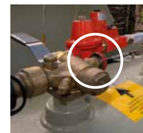
Step 1 A. Gas isolation valve - Red hand-wheel circled above
