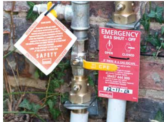
A. Emergency control valve - Closed valve
